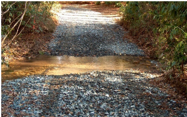
AFTER: Ample gravel applied on the approach ways. Road was widened a little to improve daylighting.
