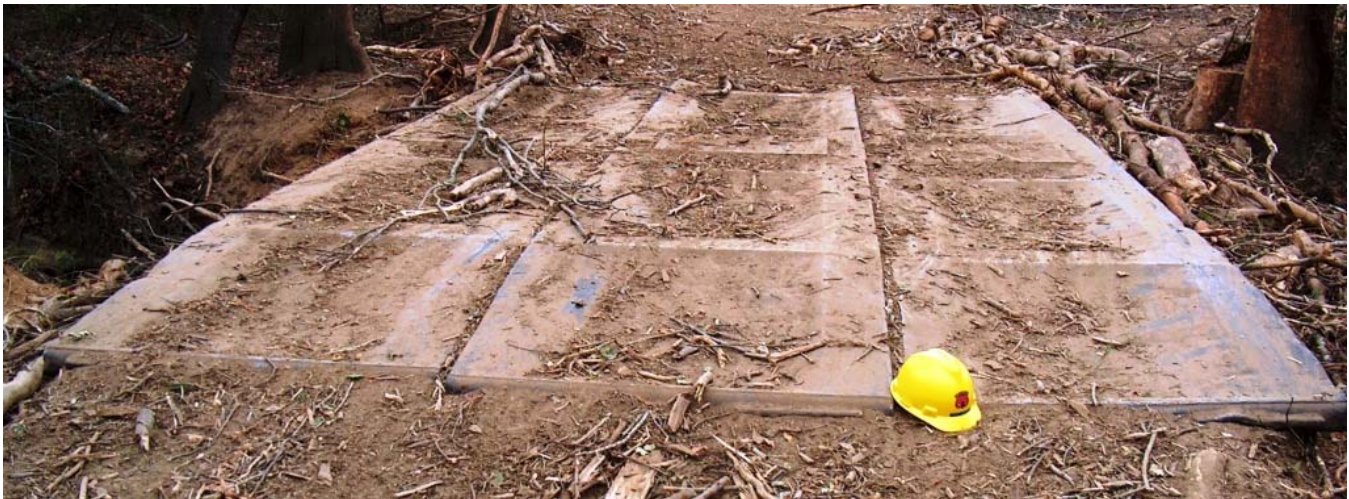
Figure 2: Gaston County, 2007. A set of NCDFR bridgemats purchased in 2003, exhibiting cupping of the 3/16-inch thick top sheeting. These bridgemats also have had steel plates welded over the center handling access holes (read below).
