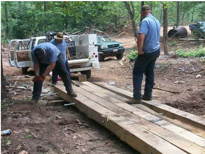
Figure 13: Alexander County, 2004. A set of wood/timber beam bridgemats being constructed in the woods by a logging company for their use.
