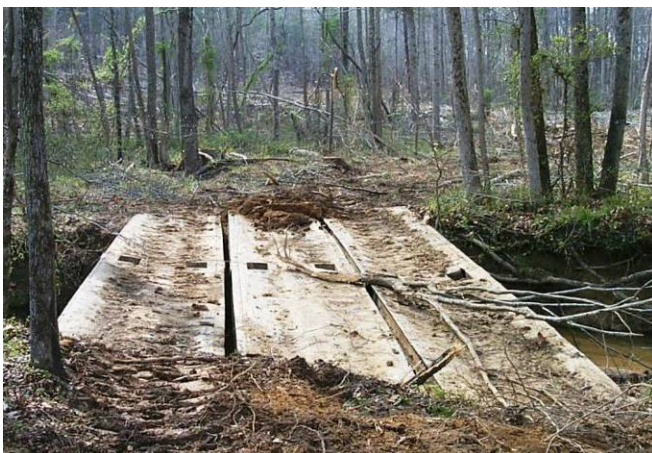
Figure 1: A set of three bridgemats installed for a skid trail crossing of a stream in central North Carolina.
