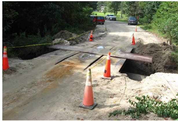
Figure 6: NCDFR bridgemats installed as temporary vehicle access for Riverbend in Moore County, NC
