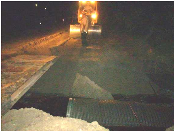
Figure 5: NCDFR personnel installing bridgemats on the same night that the road was severed from a failed culvert crossing.
