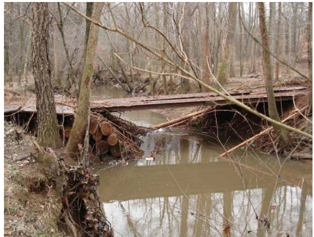
Figure 4: The logger got approval to install the two temporary log abutments in the creek channel to support the bridgemats.
