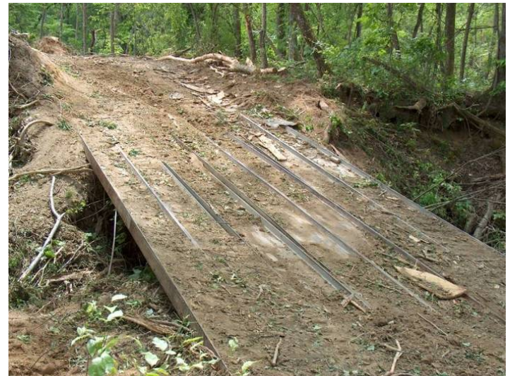
Figure 14: Iredell County, 2005. Steel I-beams are welded together to create this panel crossing. The equipment operator indicated that this panel works well for skidder crossings, but is not used at all for log trucks. Although this layout is an option, it would not appear to be a first-choice solution to constructing a bridgemat, due to potential structural and flexing issues, given the orientation of the I-beams.
