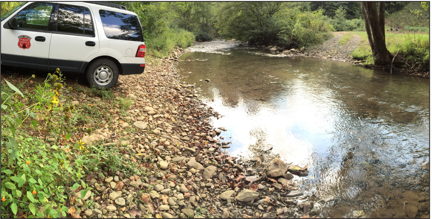
Photo 18. This is a relatively well-constructed ford crossing. The wide, stable rocky streambed and gentle approach make this a favorable location for a ford. On this harvest, the ford crossing was only used for truck access and not for skidding.
