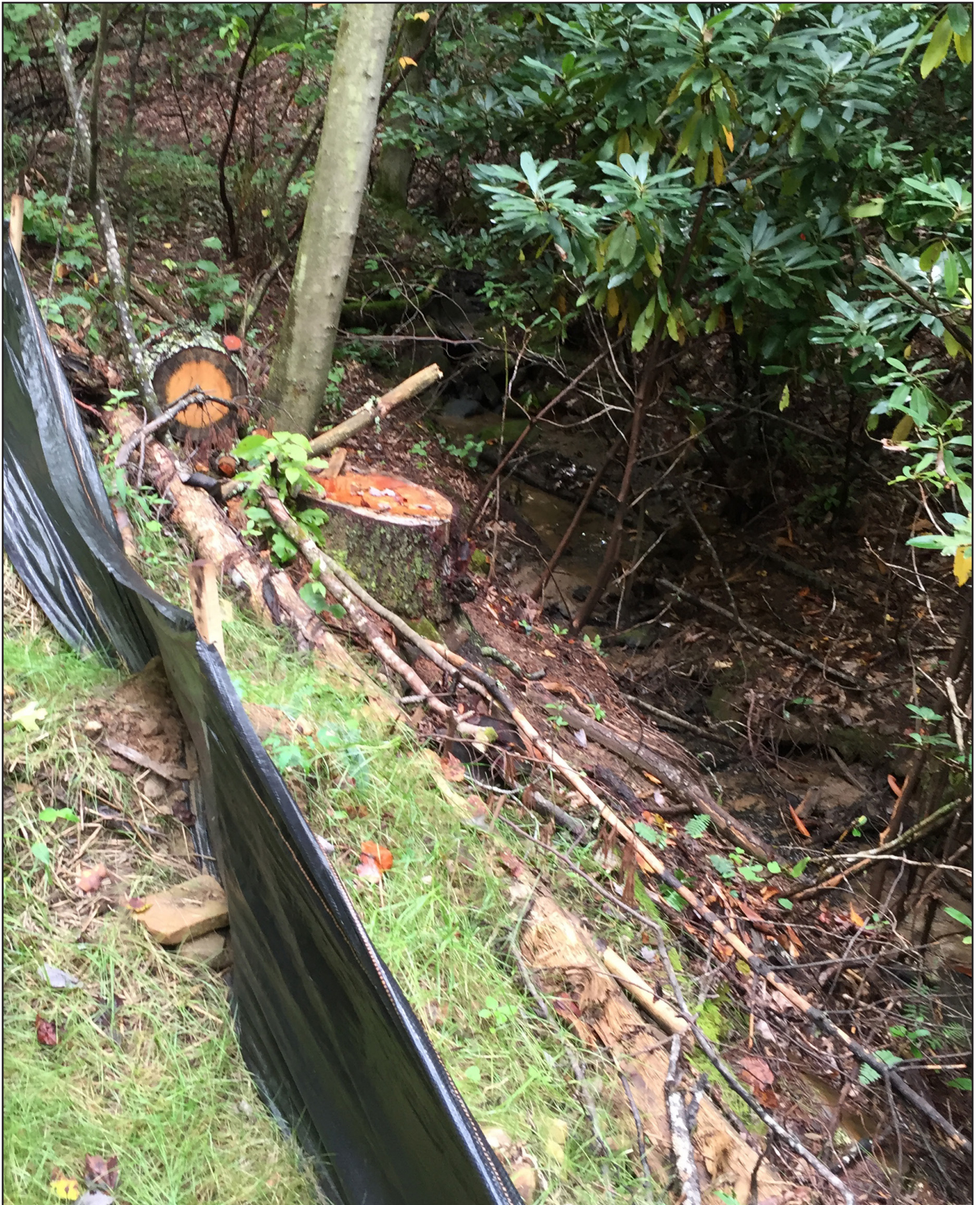
Photo 22. The forest operators installed a silt fence next to this skid trail and planted grass on the side of the trail, to prevent sediment from washing off the trail and into the SMZ. Timber was cut and removed with minimal disturbance. While this SMZ is relatively narrow, the additional BMPs that were implemented prevented visible sediment from reaching the stream.
