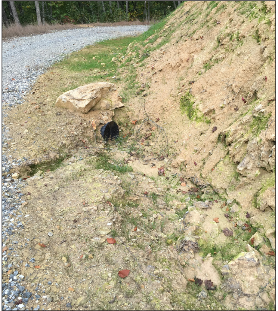
Photo 13. This cross drain collects runoff from an inside ditchline into a small pipe. The pipe runs under the road, and a brush barrier is placed under the outlet. Additionally, because the road is constructed with an inslope, water running off the road surface flows into the ditchline, and then into the cross drain. These cross drains were placed periodically down the length of the road, to prevent runoff from accumulating and overwhelming a single drain. The ditchline in this photo needed stabilization work to reduce erosion and sedimentation.
