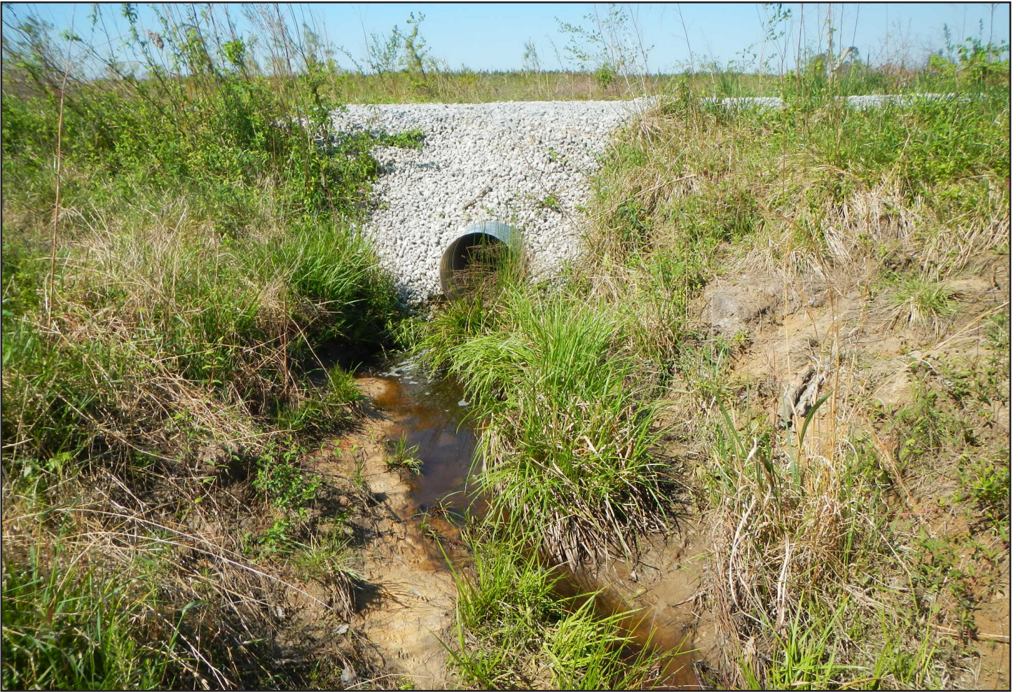
Photo 16. This culvert headwall was well stabilized, and the culvert appears large enough to handle water flow. Vegetation has been maintained on the streambanks and above the culvert, and the road above the crossing receives plenty of daylight, all measures that can help to limit erosion.
