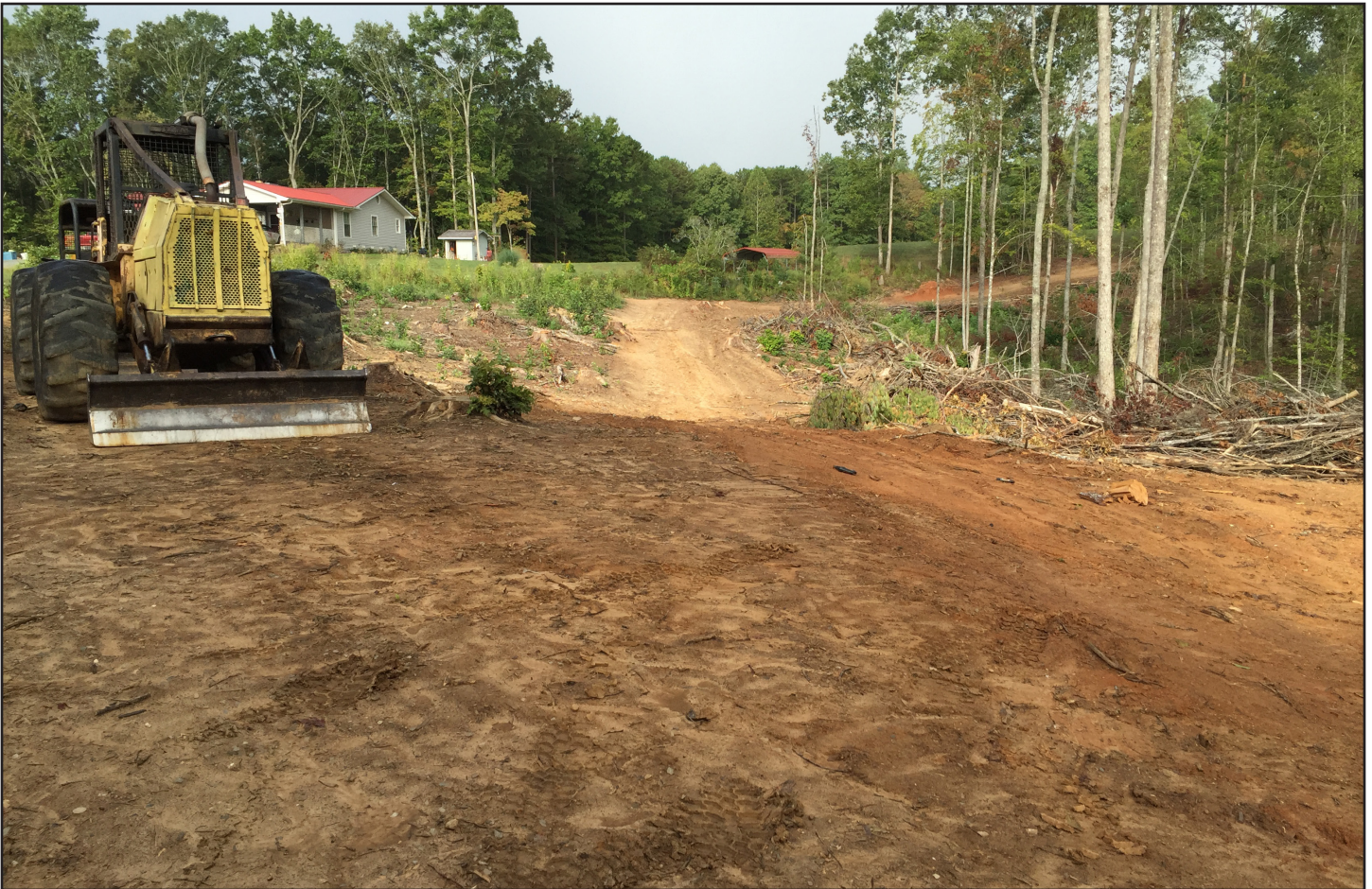
Photo 4. On this site in the Mountains, the deck is situated on a flat area near the top of a ridge, and a brush barrier on the right side of the picture helps to prevent sediment from traveling downslope into a ravine. However, more logging debris could be placed on the deck and the skid trail in the background, to further limit soil disturbance and erosion.
