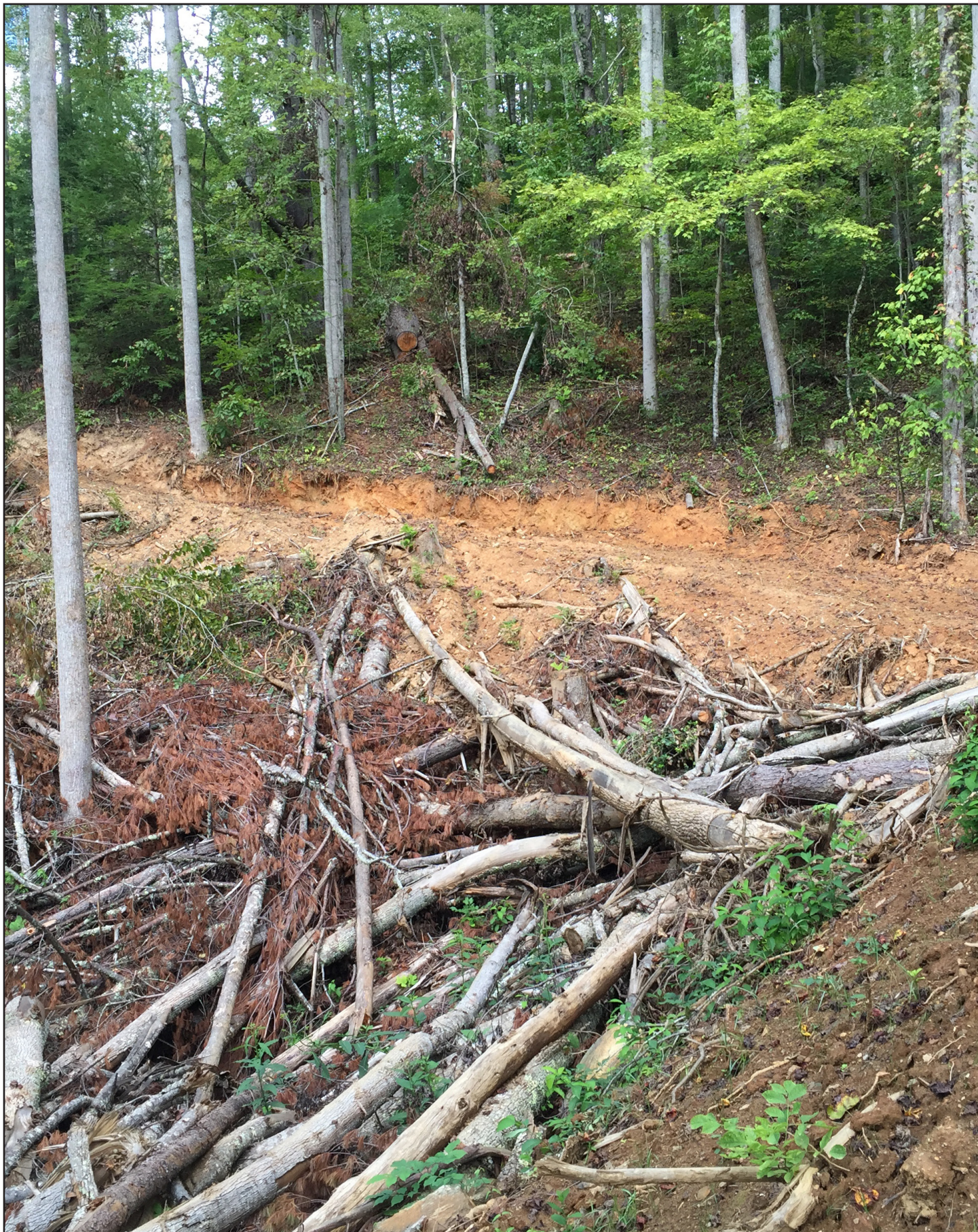
Photo 3. At this site, the forest operator placed logging debris along the edge of a skid trail to prevent sediment from traveling downslope. However, sediment movement could be prevented further by placing some of that debris atop of the skid trail itself.
