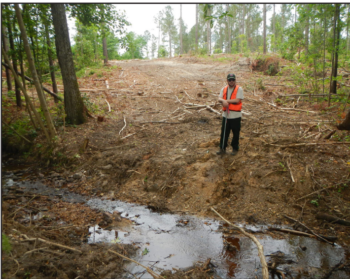
Photo 9. Stream crossing that was removed and still in need of BMP stabilization.
