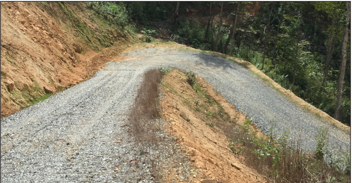
Photo 14. Example of a switchback on a steep mountain road. Gravel was applied to stabilize the surface. Additional BMP work should occur on the exposed soil of the cut banks.
