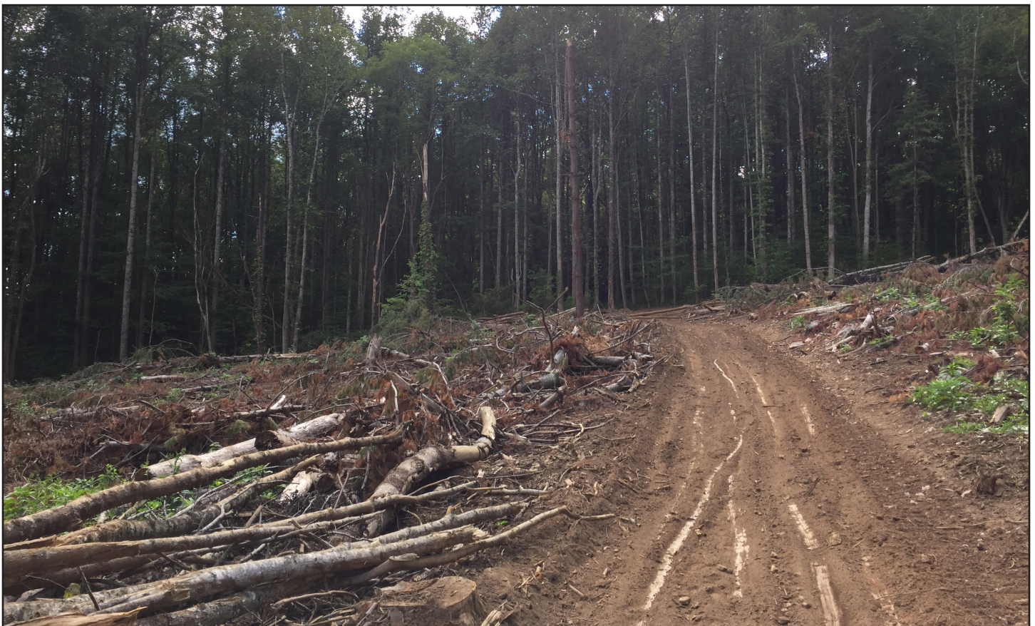
Photo 12. This skid trail generally follows the contours of the land, which helps to limit the slope of any skid trail segments. However, the leftover logging debris could be placed on top of the trail to prevent erosion and runoff.
