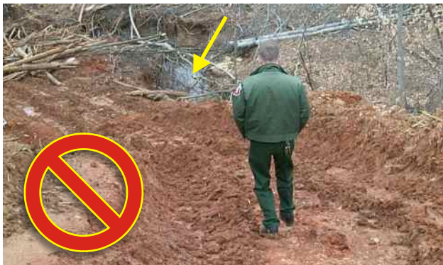
Rutted and unstable soil on a skid trail leading toward the stream. Also, no SMZ was left along the stream (arrow).
