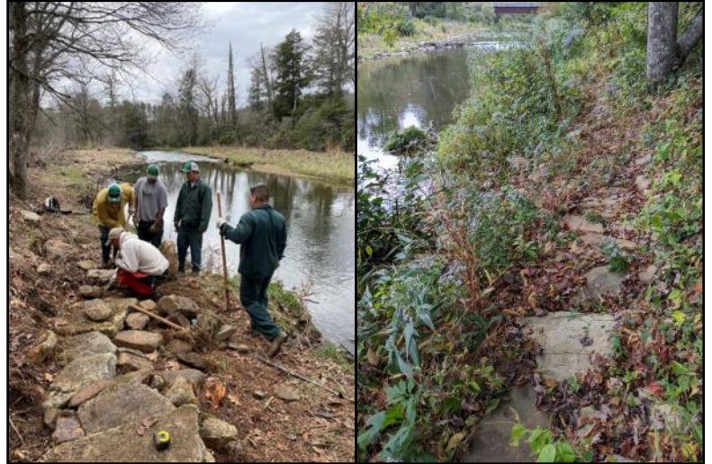
NCFS B.R.I.D.G.E crew installing stones for the fishing trail (left) and a photo of an installed section of trail taken a couple of months later (right).
